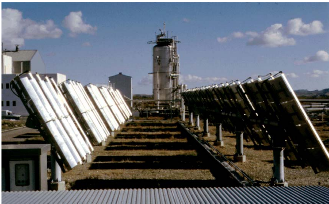
Figure 3.4b View of all the Pilot Plant in operation
