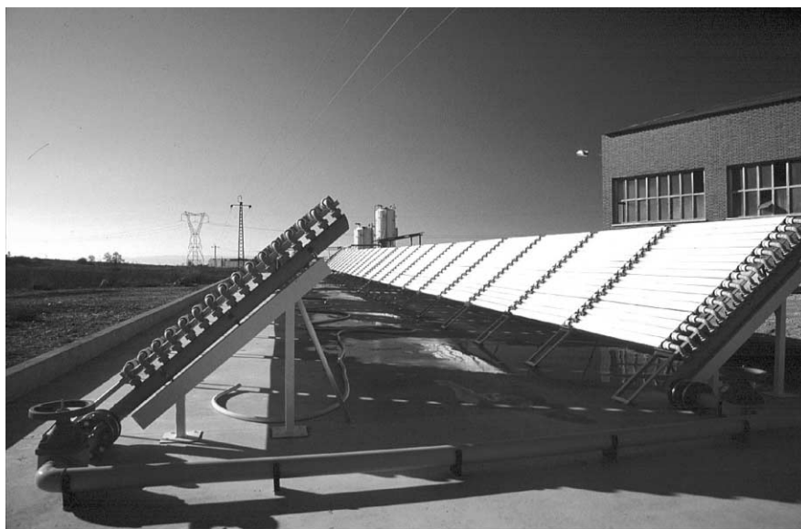
Fig. 3. Partial view of the demonstration plant based on CPCs.
