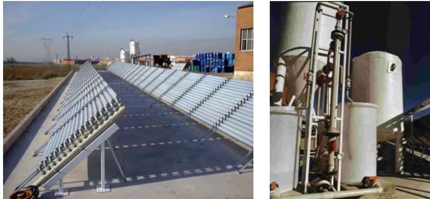
Figure 3.4. Images of the photoreactor (left) and the \text{TiO}_2 recovery system (right) of Hidrocen solar detoxification plant.
