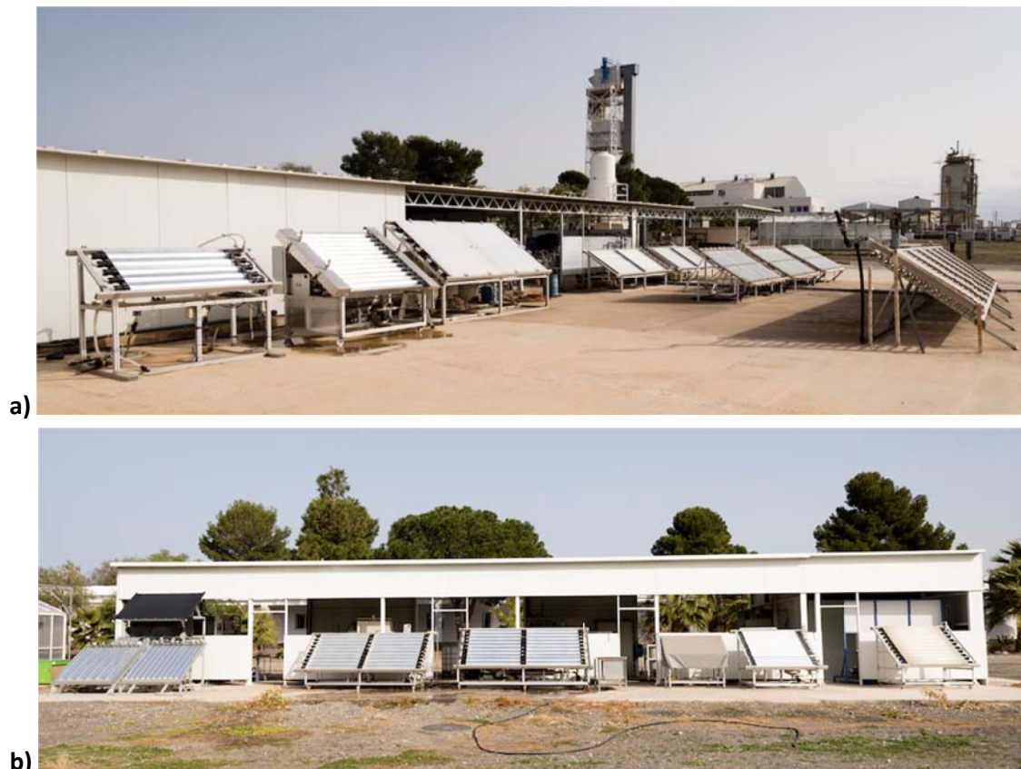
Figure 58. View of several CPC photo-reactors for purification of water. a) CPC facilities I, b) CPC facilities II.
