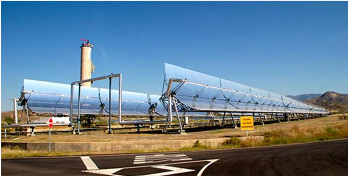
Figure 11. View of the DISS plant solar field in operation
