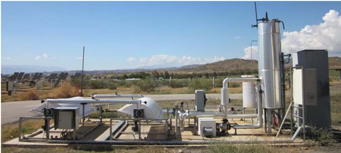
Figure 17. CAPSOL solar thermal test facility for small-size parabolic-trough collectors.
