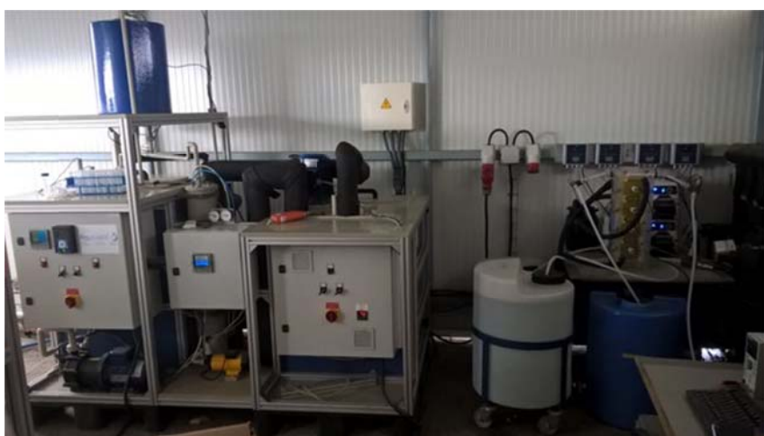
Figure 95. Pilot-plant for assessment of combined reverse electrodialysis and membrane distillation
