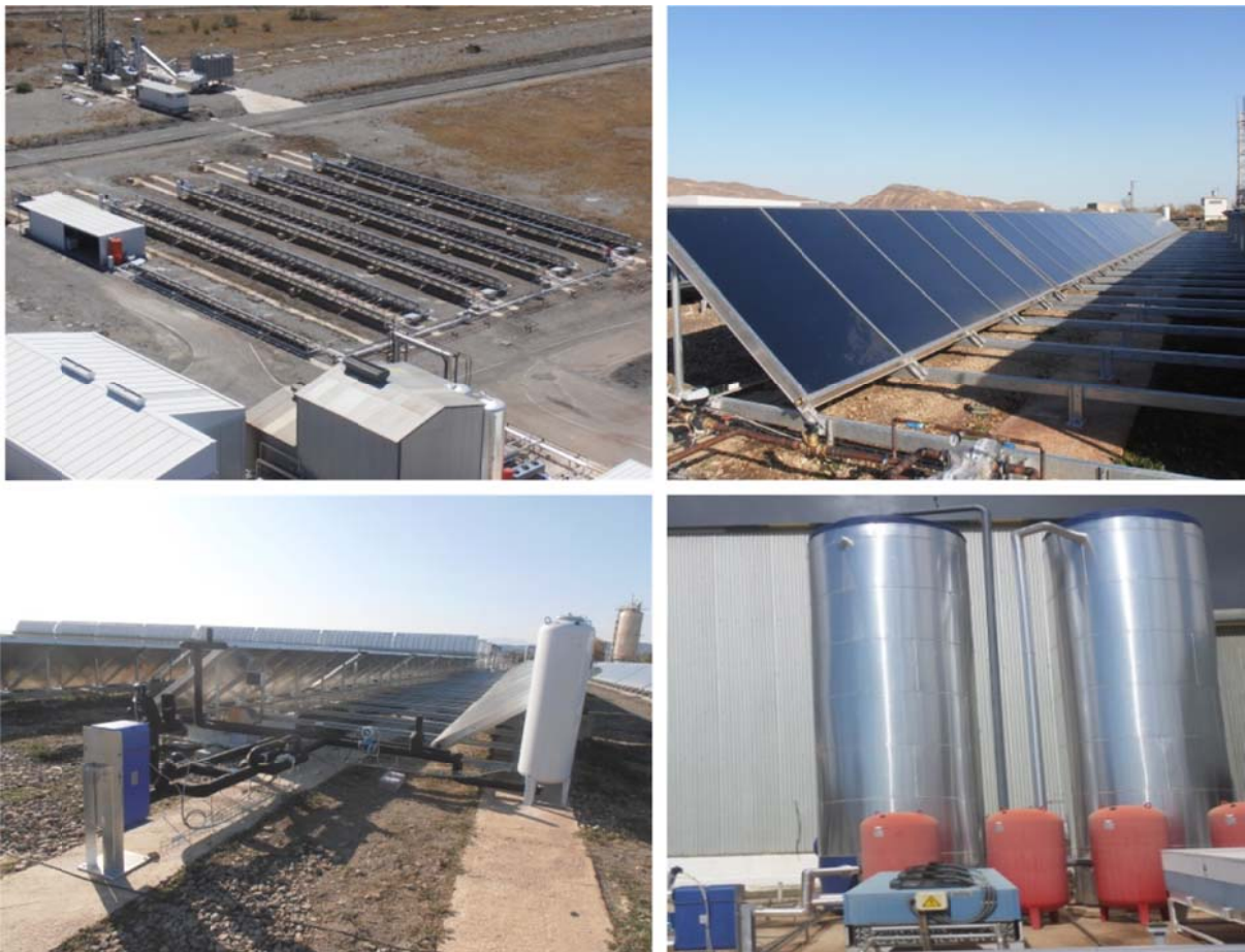
Figure 30. The 606-m 2 large-aperture flat plate solar collector field (AQUASOL-II)
