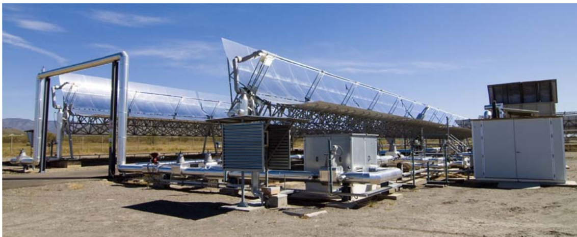
Figure 12. View of the IFL experimental facility (with parabolic-troughs) using compressed gas as heat transfer fluid.
