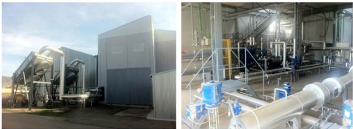
Figure 31. View of the outside of the CSP+D test bed building with the air coolers (left) and partial view of the interior of the CSP+D test bench (right)
