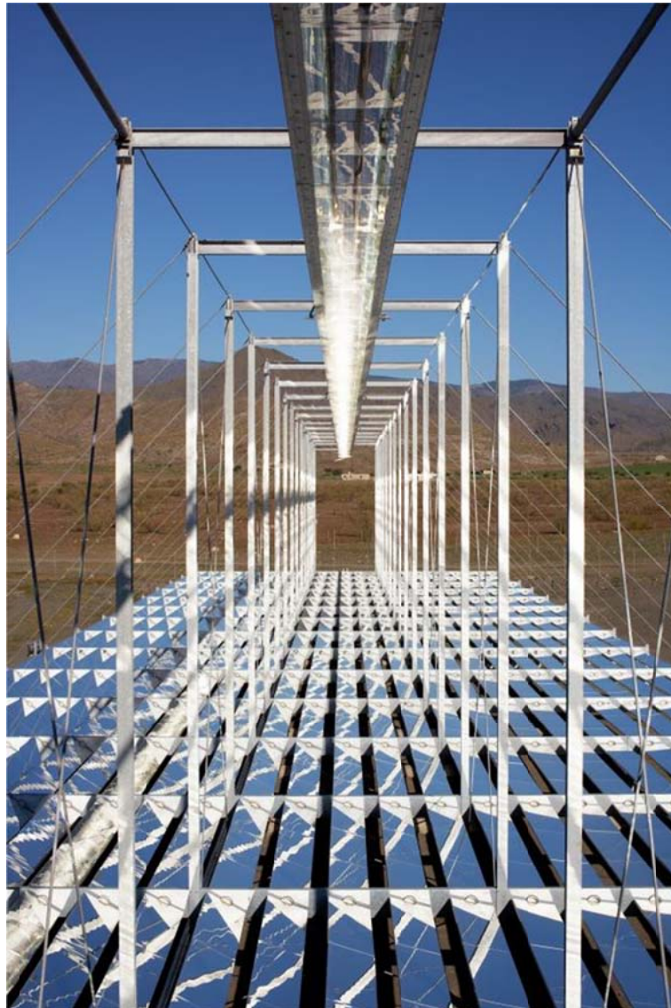
Figure 16. Photo of the linear Fresnel concentrator erected at the PSA.
