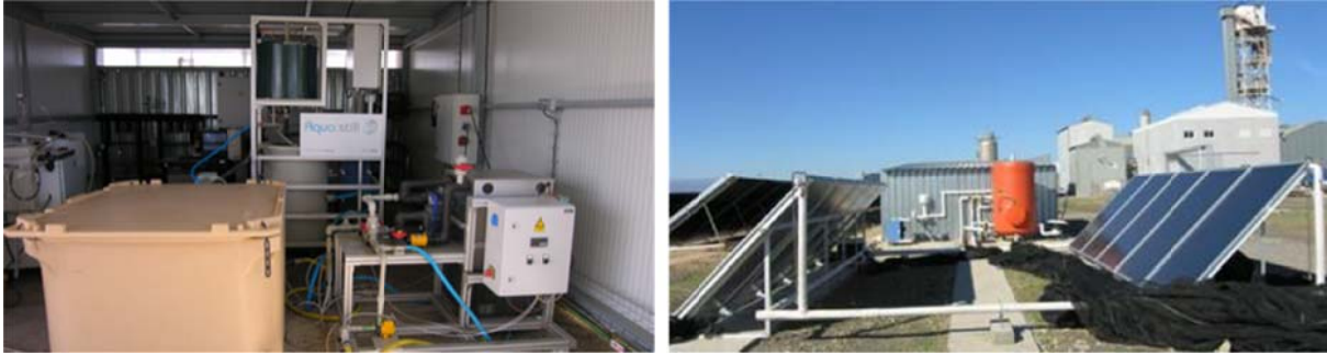
Figure 33. Internal (left) and external (right) views of the Membrane Distillation experimental test bed within the PSA low-temperature solar thermal desalination facility.
