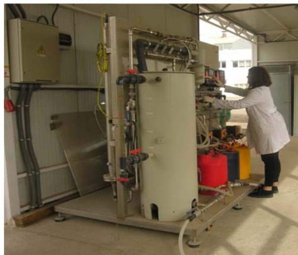
Figure 64. UVC pilot plant installed at PSA facilities.
