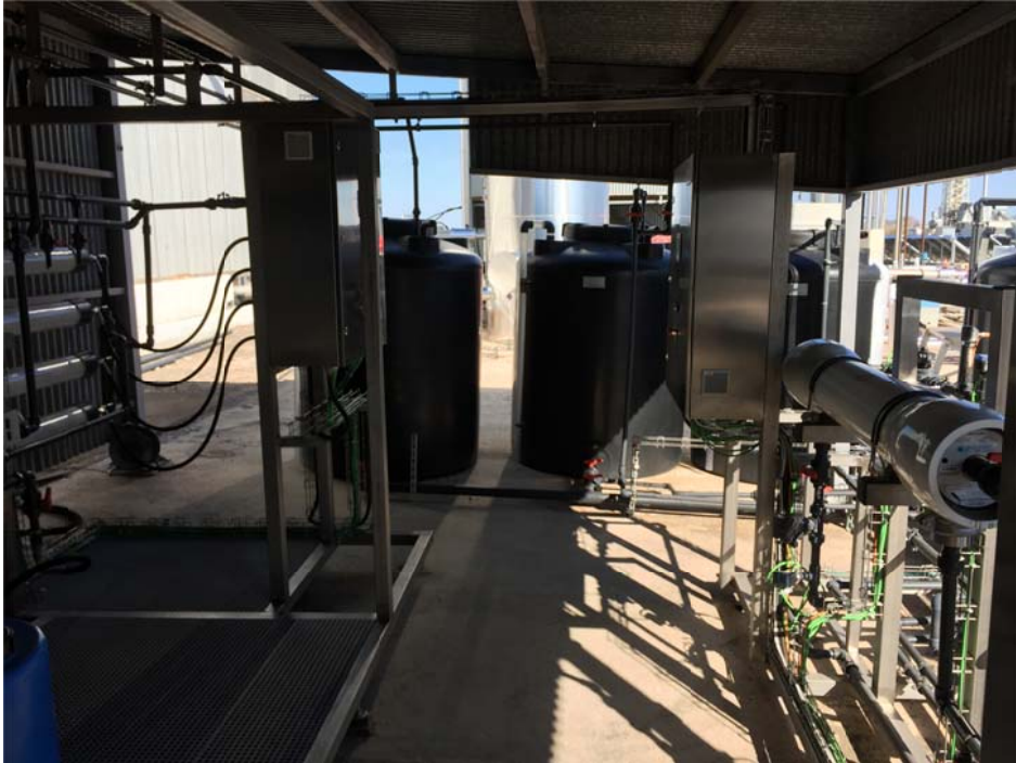
Figure 37. Test bed for FO-RO combination research
