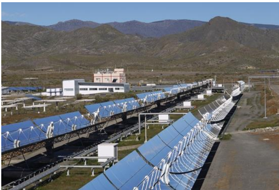
Figure 3.6: View of the DISS test facility including Solarlite's SL4600 collectors installed for the DUKE project.
