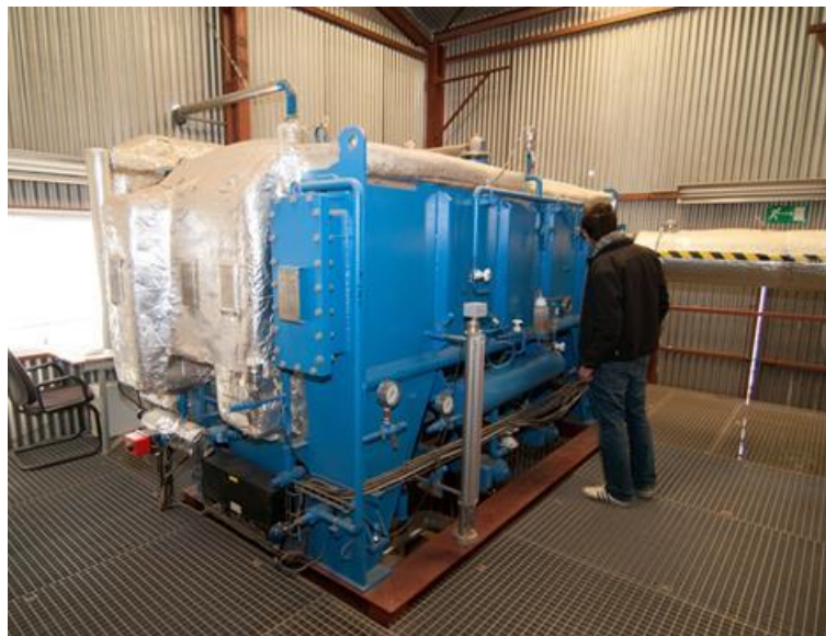
Figure 6.5. Picture of the absorption heat pump in AQUASOL facility.
