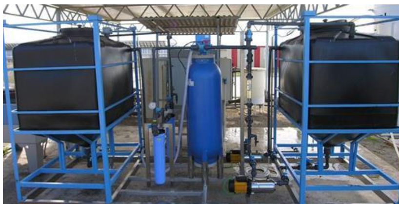
Figure 2.40. Filtration/flocculation pilot plant for treating raw water.
