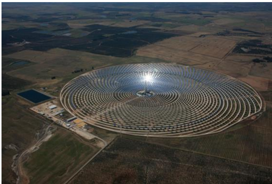
Figure 3.13. Aerial view of GEMASOLAR plant under operation
