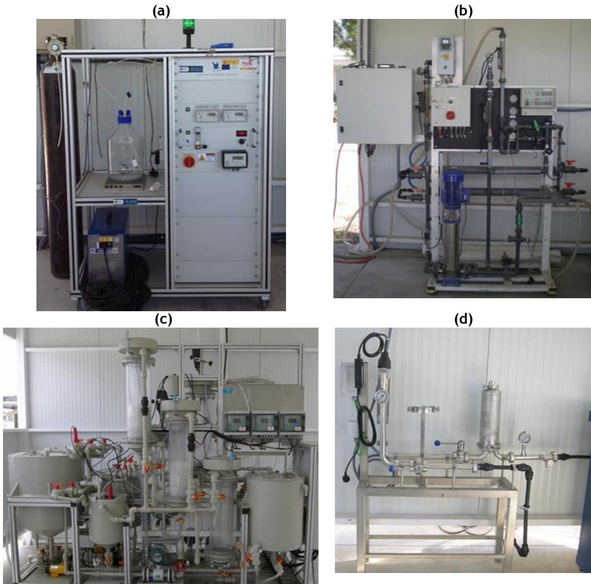
Figure 2.39. New pilot plants located in the new hangar: Ozonation (a), Nanofiltration (b), Biologic system (c) and disinfection UV/filtration (d).
