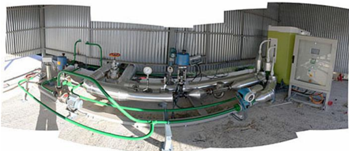
Figure 2.34. Solar ORC experimental facility
