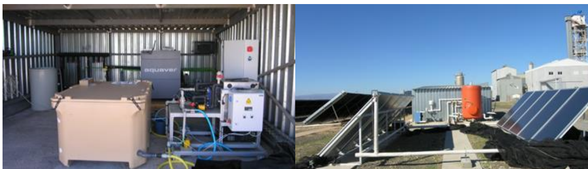
Figure 2.35. Internal (left) and external (right) views of the Membrane Distillation experimental test bed within the PSA low-temperature solar thermal desalination facility
